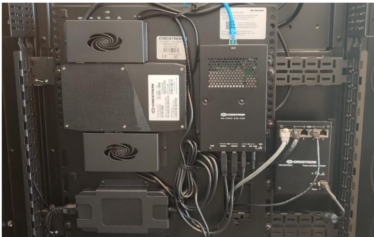
Figure 2: Crestron Flex R-Series – Rear Equipment Rack including the UC Engine Assembly
