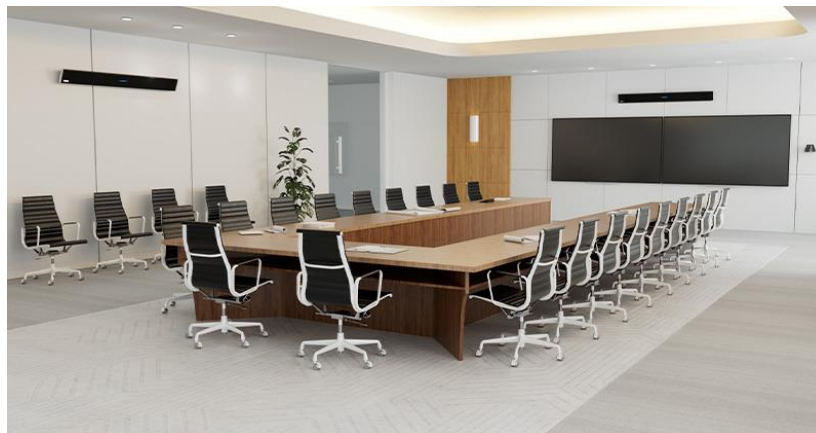
Figure 5 – Nureva HDL Devices Installed in a Meeting Room
